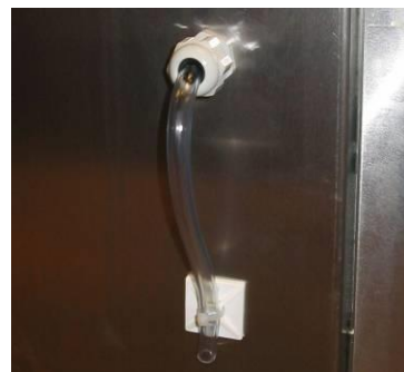
Figure 2. Mounting of pressure hose for measuring of atmospheric pressure.
