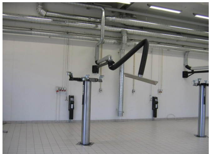
Workshop Environment with Panel fume extractor
