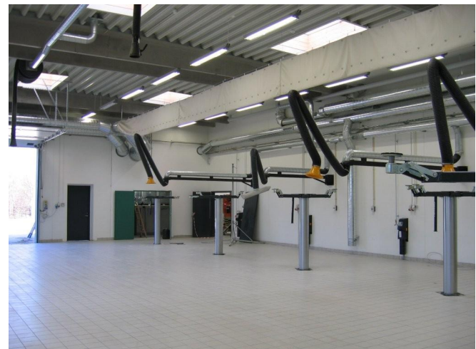
Workshop Environment with Panel fume extractor
