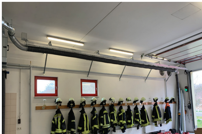
MRSP installed in a German fire station
